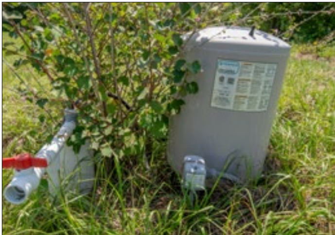
New 5-inch well with 1.5 HP submersible pump
